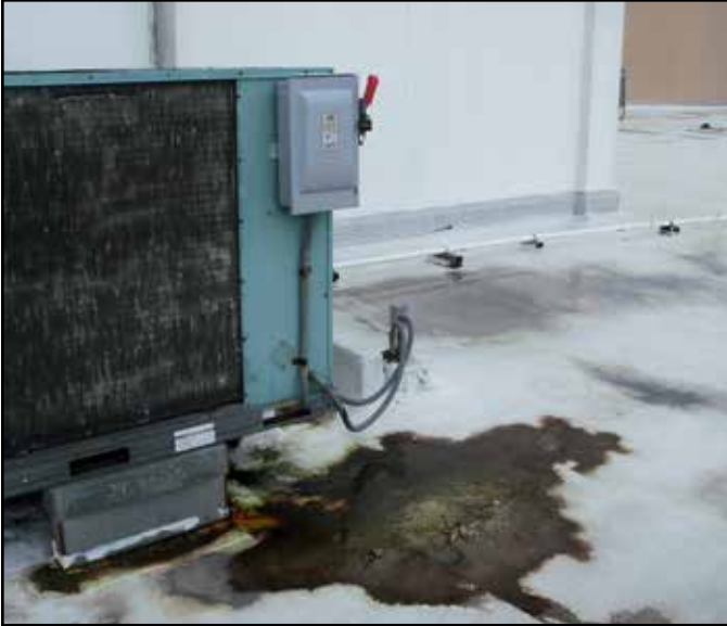
Disconnected condensate drain lines
