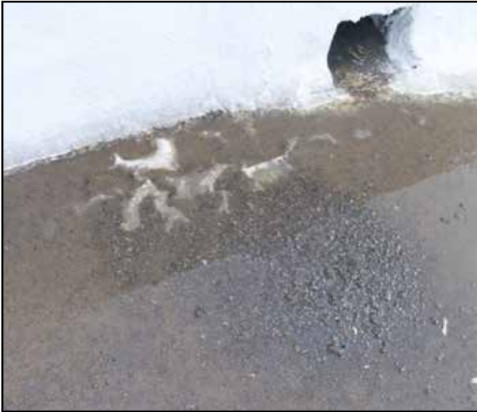
Scupper installed too high
