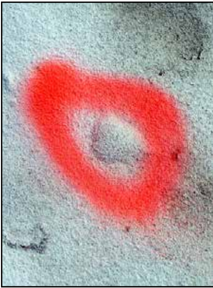
Blister due to contamination
