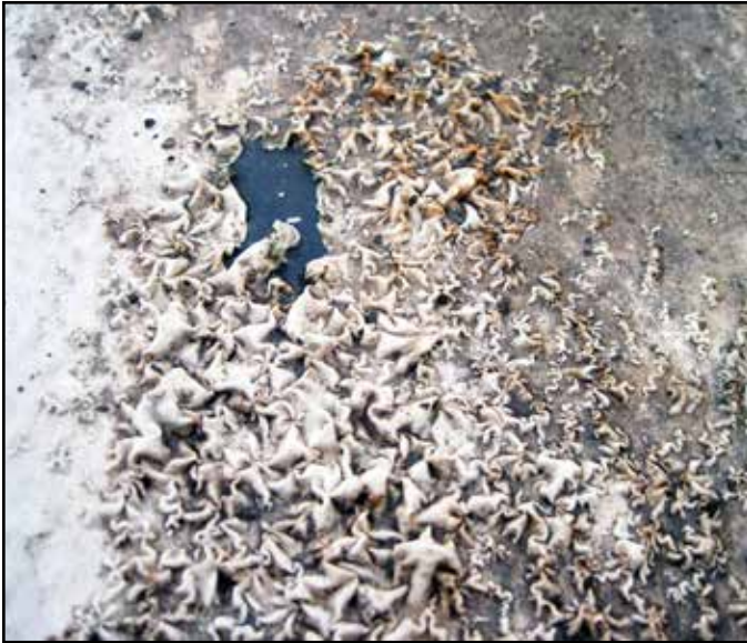
Delamination due to thin topcoat and ponding
