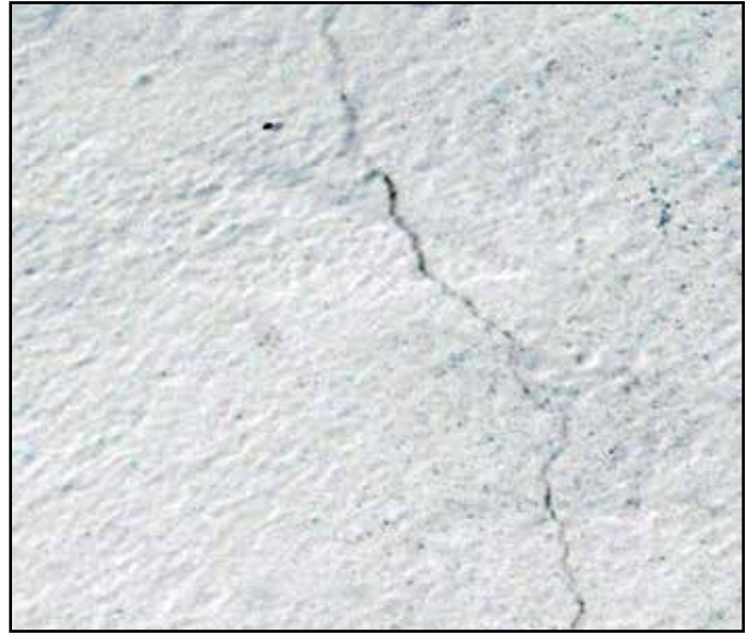
Crack in coating telegraphed from concrete
