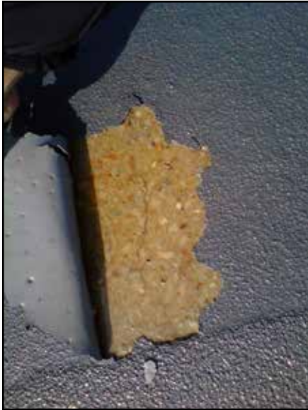
Delamination due to moisture
