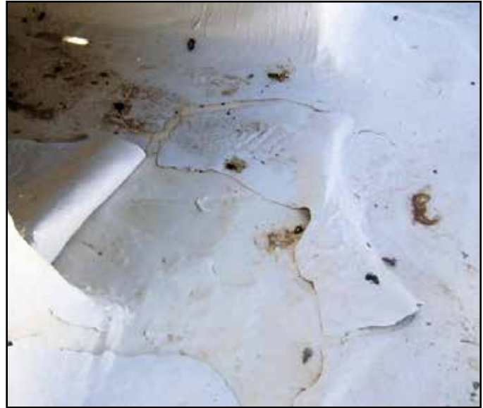
Delamination due to improper cleaning
