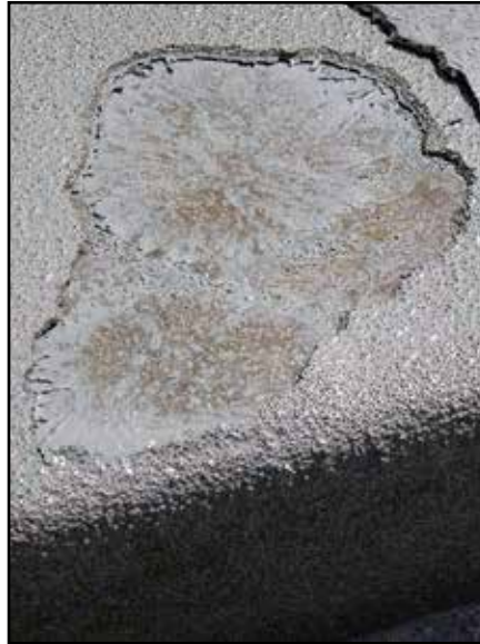
Area underneath removed blister
