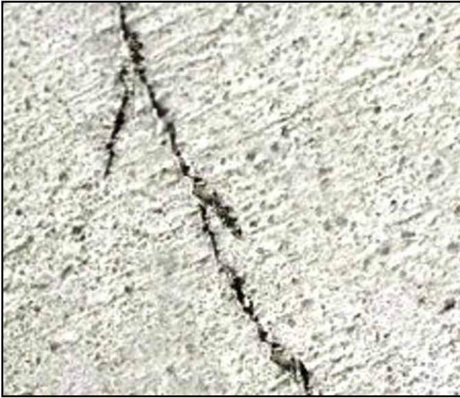
Crack before coating
