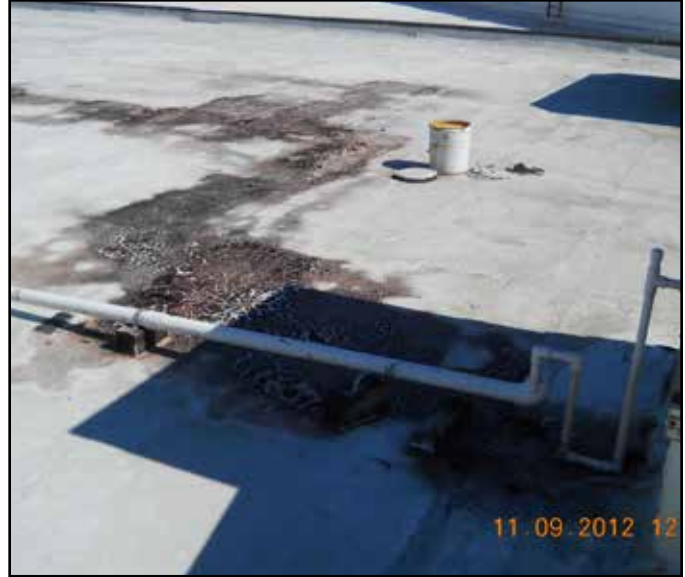
Poorly maintained condensate drain lines
