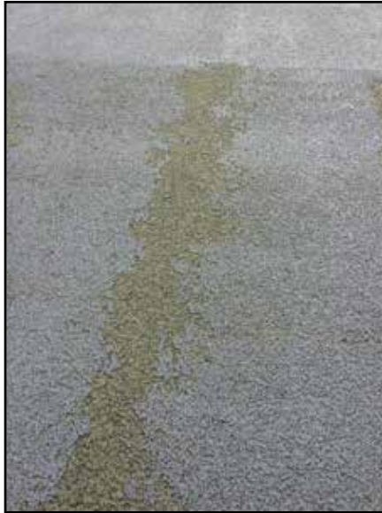
Delamination due to incompatible materials
