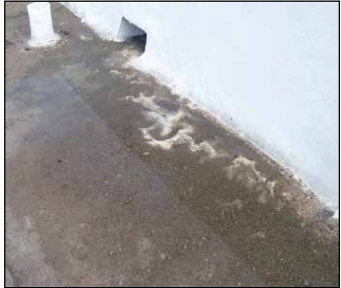
Clogged roof drain
