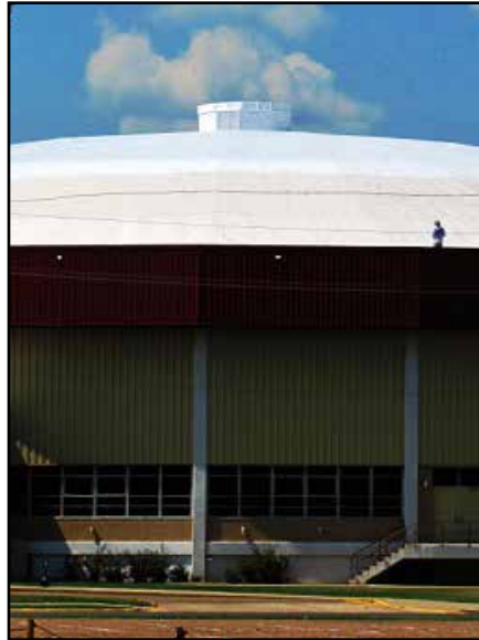
Roof with moisture contamination
